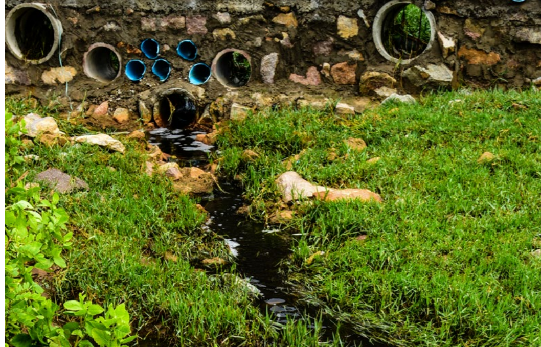
Effluent outlet pipes behind Ramky Hazardous Waste Plant
